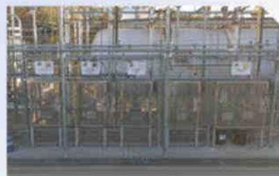
AFTER: New unloading portals with magnetic key fob access (photo courtesy of MGPI)
