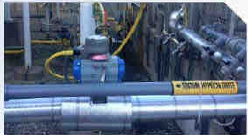
New shutoff valve (photo courtesy of MGPI)
